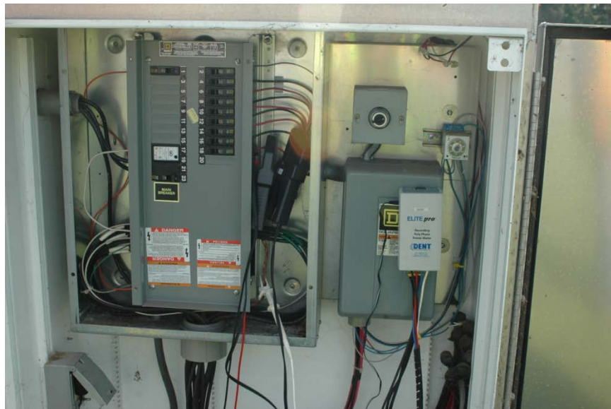
Clem's Way panel located on the southwest corner of Business Park Dr. and Clem's Way. Circuits 16 & 18 were measured
