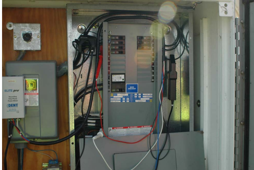
E.M. Copps Dr. panels located on the northeast corner of E.M. Copps Dr. and Weeks St. Circuits 5 & 6 were measured
